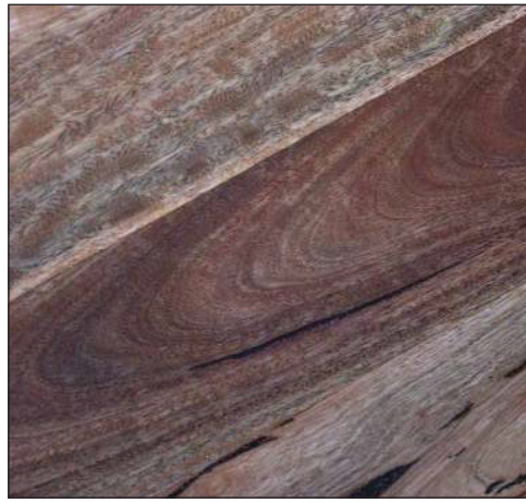
The photo to the left shows circular swirl marks that are visible under down light. The photo to the right shows the same section of floor in natural light without the down lights on and the swirl marks are not visible.
